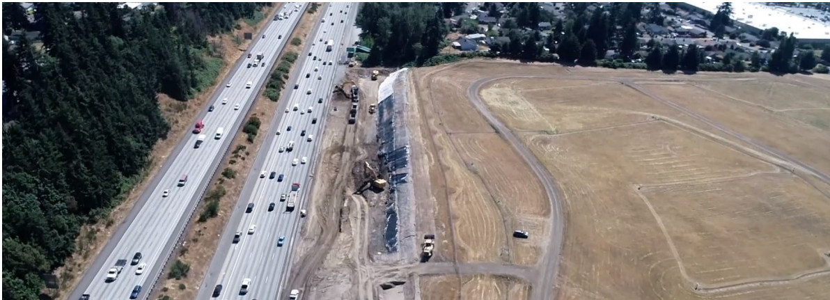
Midway Landfill waste removal project, which will restore remedial action components and provide space to add two lanes to Interstate 5 and build the Federal Way Link Light Rail Guideway (Source: Jeff Neuner and Kiewit Corporation)
