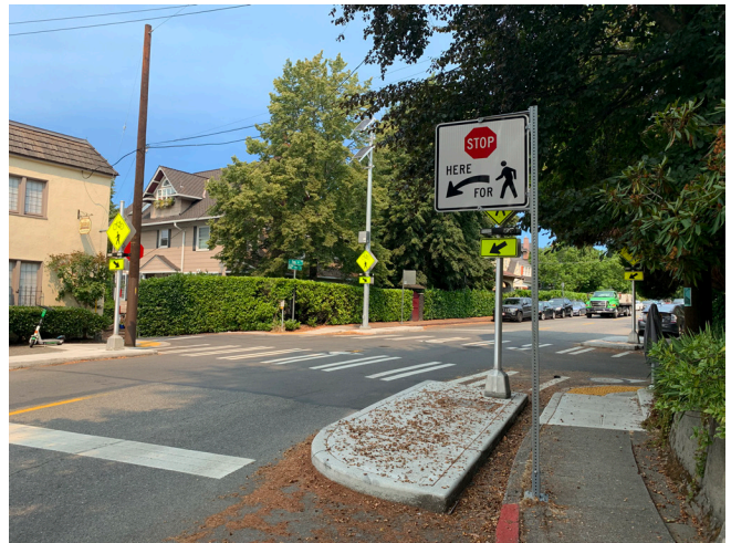
Crossing improvement at 12th Ave E and E Roy St as part of the Lowell Meany Neighborhood Greenway Project
