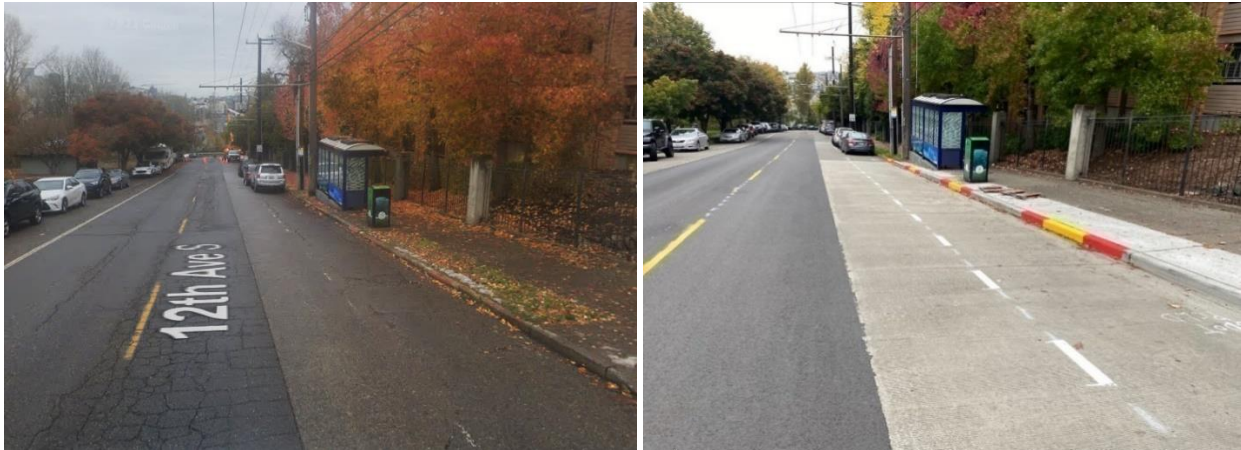
Program 21 – Before (left) and after (right) pavement repair and bus stop improvements on 12th Ave S and S Judkins St in North Beacon Hill, as part of a partnership with Program 9 - Paving Spot Improvements .
