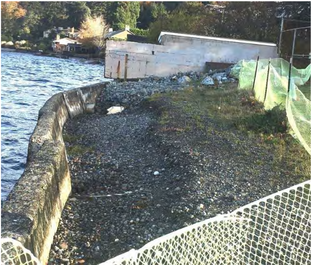
Figure 1. Failed Seawall (Photo taken on 10/18/2016).
