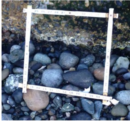
A. Private seawall toe cobble north of park
