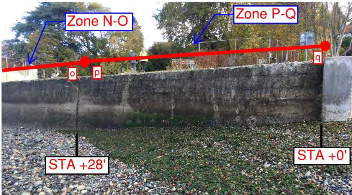
Photo 2. South Portion of Seawall. Source: Reid Middleton Site Visit 10/18/2016 Note: Dimensions roughly field measured – for assessment purposes only.
