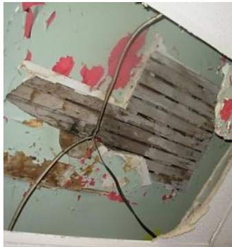
Housing code violations at Sisley rental houses
