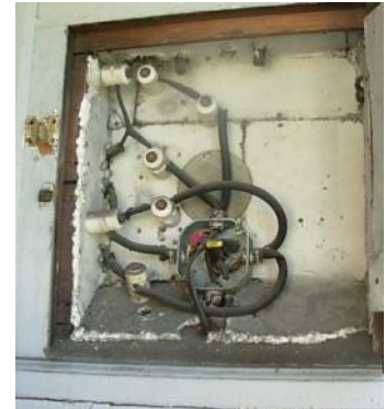
Housing code violations at Sisley rental houses
