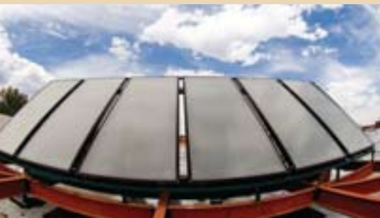
Solar water heating at REI.
