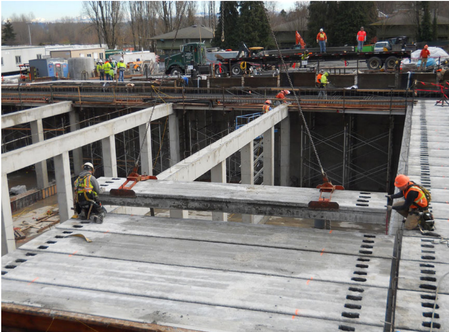
Construction of a storage tank in the Windermere neighborhood that will capture sewage and stormwater during heavy rains.
