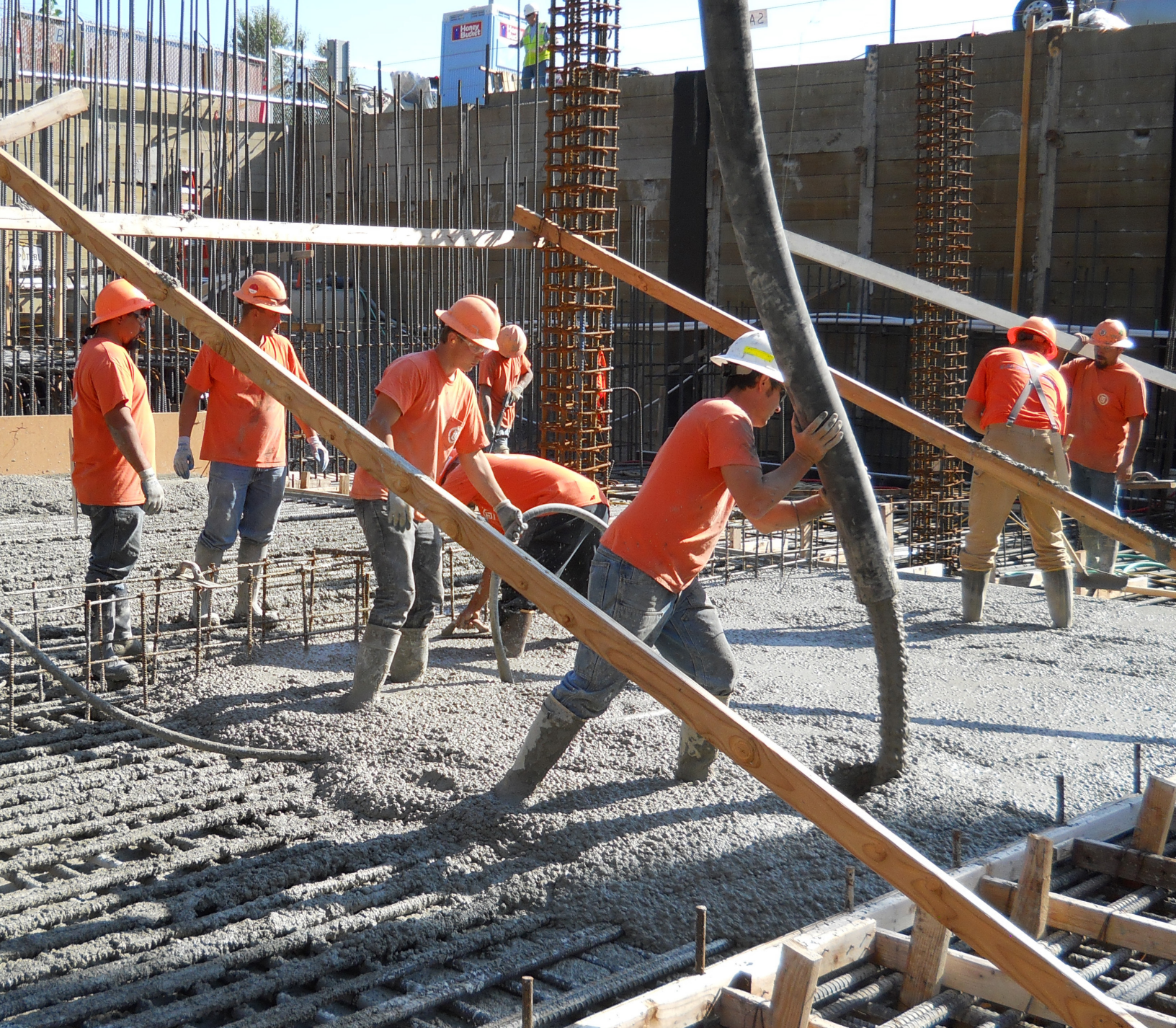
Pouring the foundation for a 2-million-gallon storage tank to keep pollution from reaching Lake Washington.
