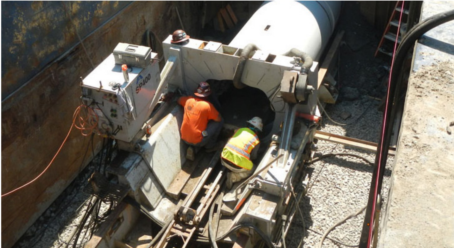
Installing a new section of pipe for the Madison Valley Stormwater Project.
