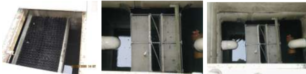
Oil/Water Separator (coalescing plate)
