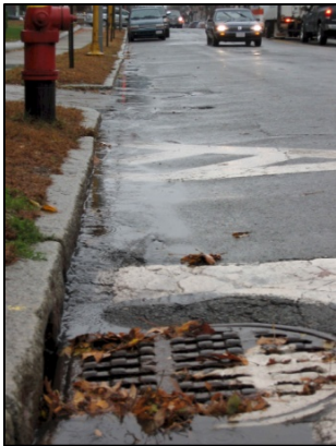
Stormwater Runoff to Streets
