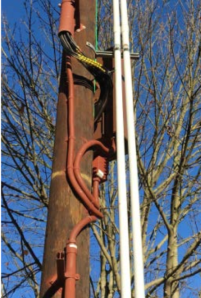
Figure 8 Example of unallowed excessive bends in flex conduit
