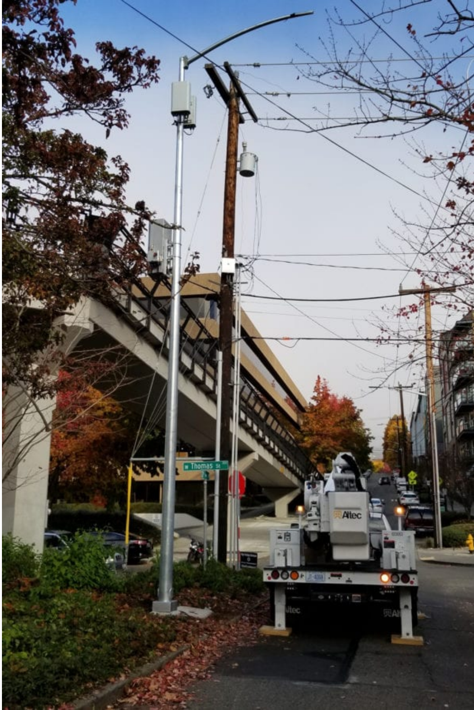
Figure 9 Metal pole with side-mount panel antennas and equipment cabinet
