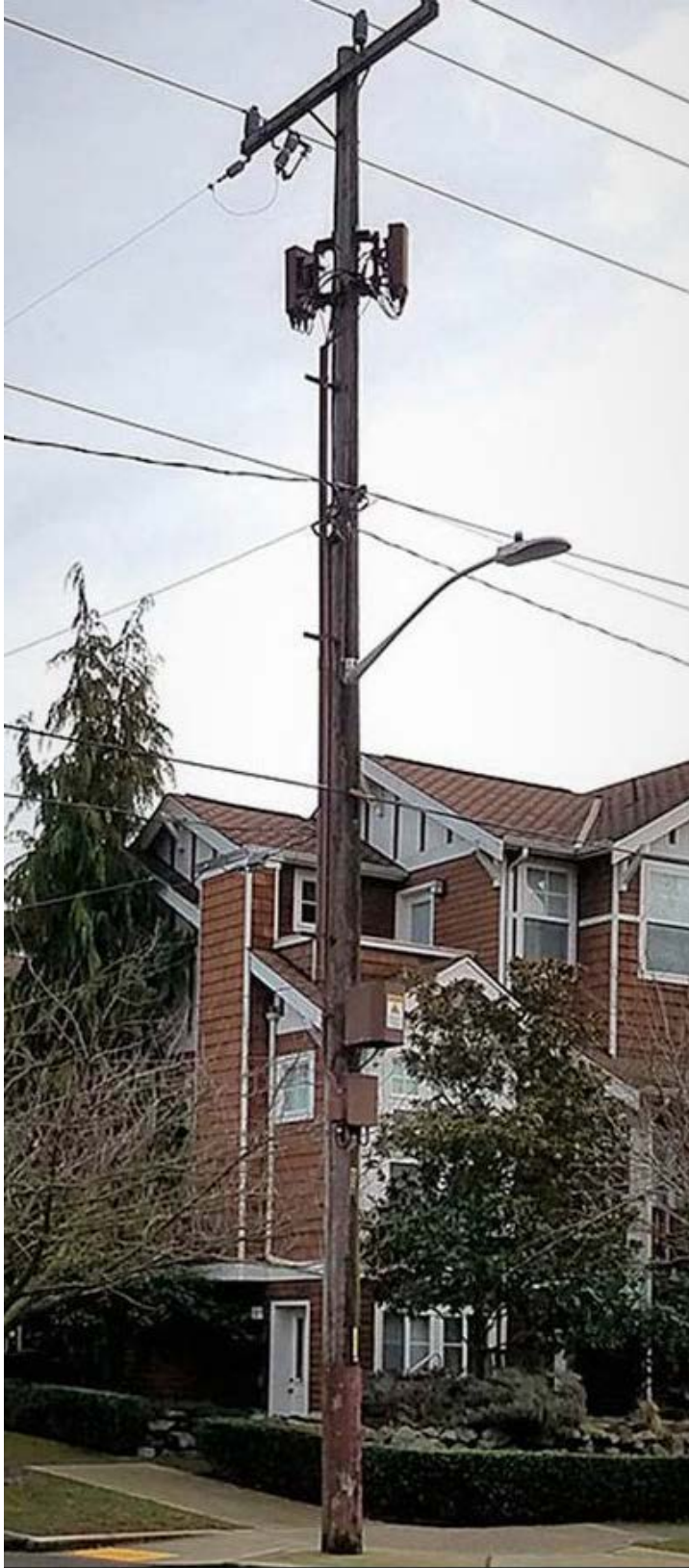
Figure 6 Typical wood pole design with panel antennas
